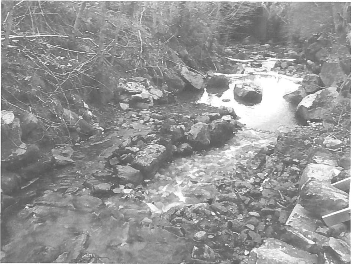
Photograph of the structure (downstream view) taken after the easement works (under low flow conditions)
